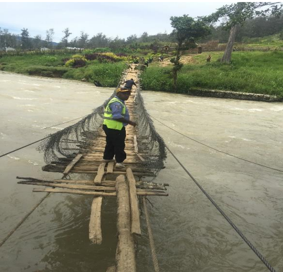
Figure 7. Team Leader on a bridge connected by one log.
